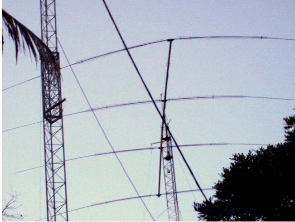
Arcing in broken linear-loading tubes
